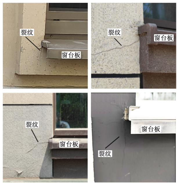
图3 窗角部位外墙外保温系统面层砂浆开裂 Fig.3 Mortar cracking on the surface of external wall external insulation system at the window corner
