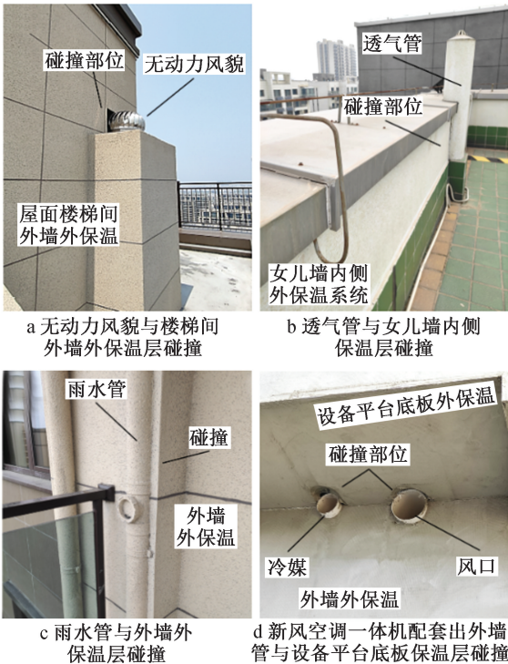
图 1 各类管线与保温层碰撞现场 Fig.1 Collision between various pipelines and insulation layer
