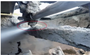
图 2 喷洒梁雾化喷水系统 Fig.2 Spray beam atomizing water system
